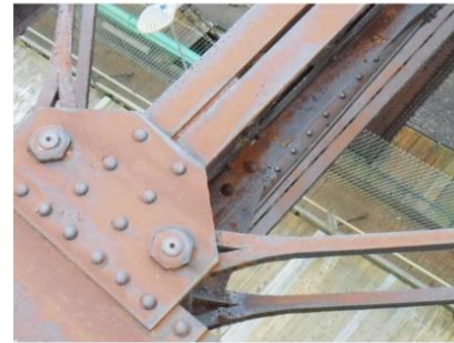
North Bay – U14 Sway Brace
