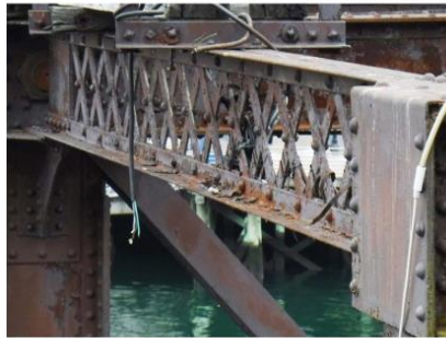
Center Bay – U22 Sway Brace
