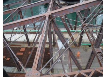
South Bay – U14 Sway Brace
